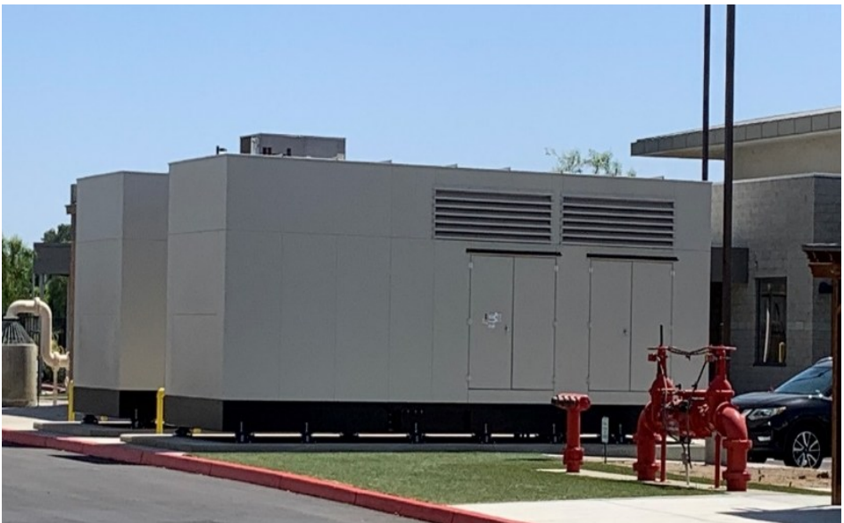
Emergency Backup Generators at YLWD Headquarters
