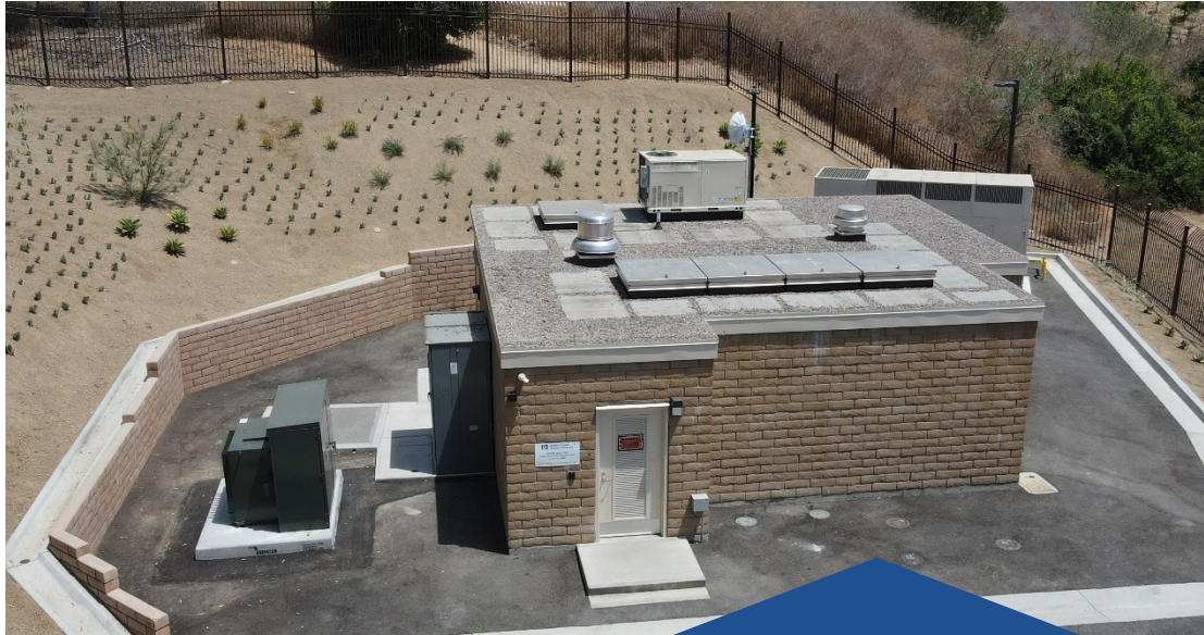
Hidden Hills B.P.S. Design Pumping Capacity: 3,600 GPM
