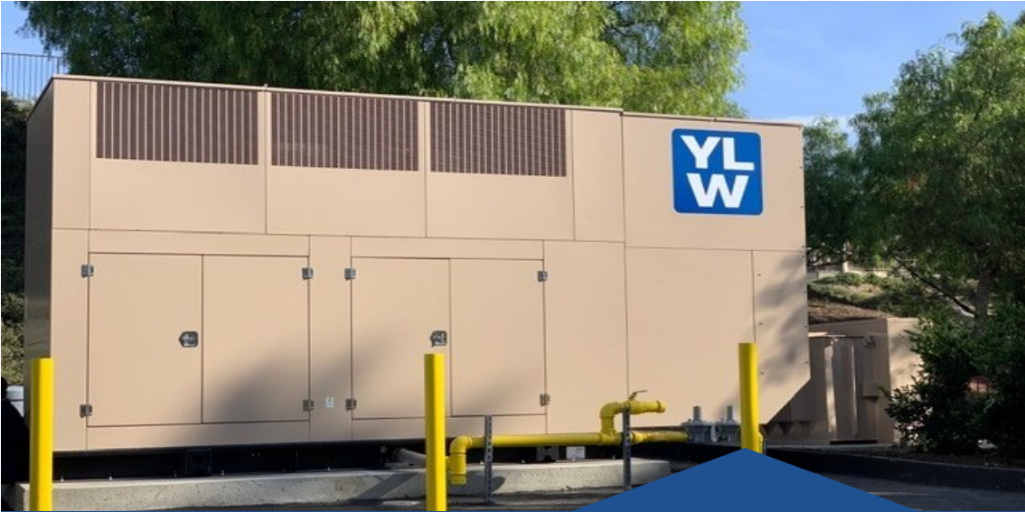
Elk Mountain Emergency Backup Generator – 500kw Elevation: 780'
