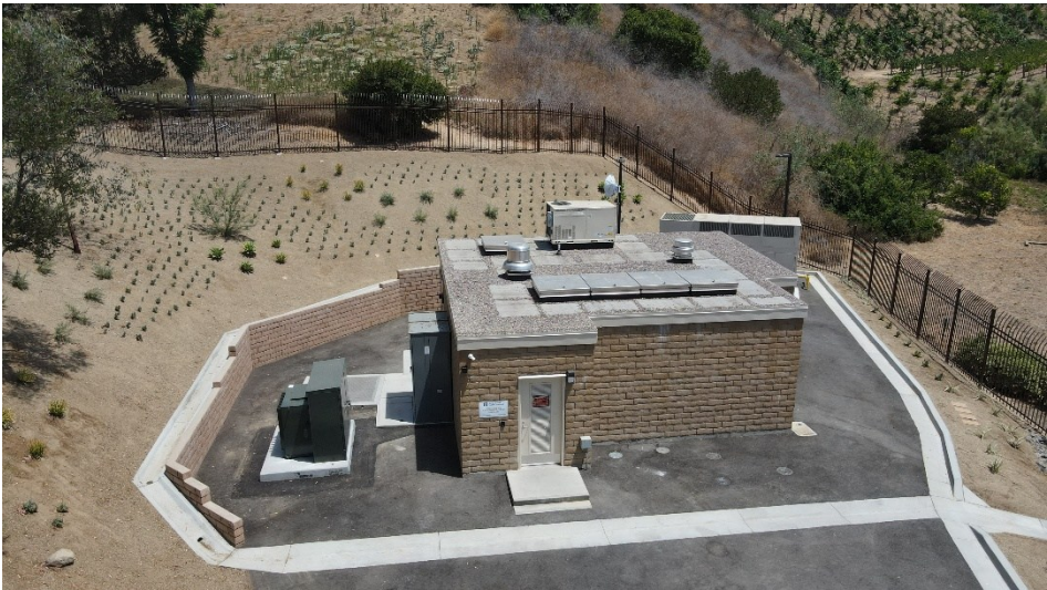
Hidden Hills Booster Pump Station
