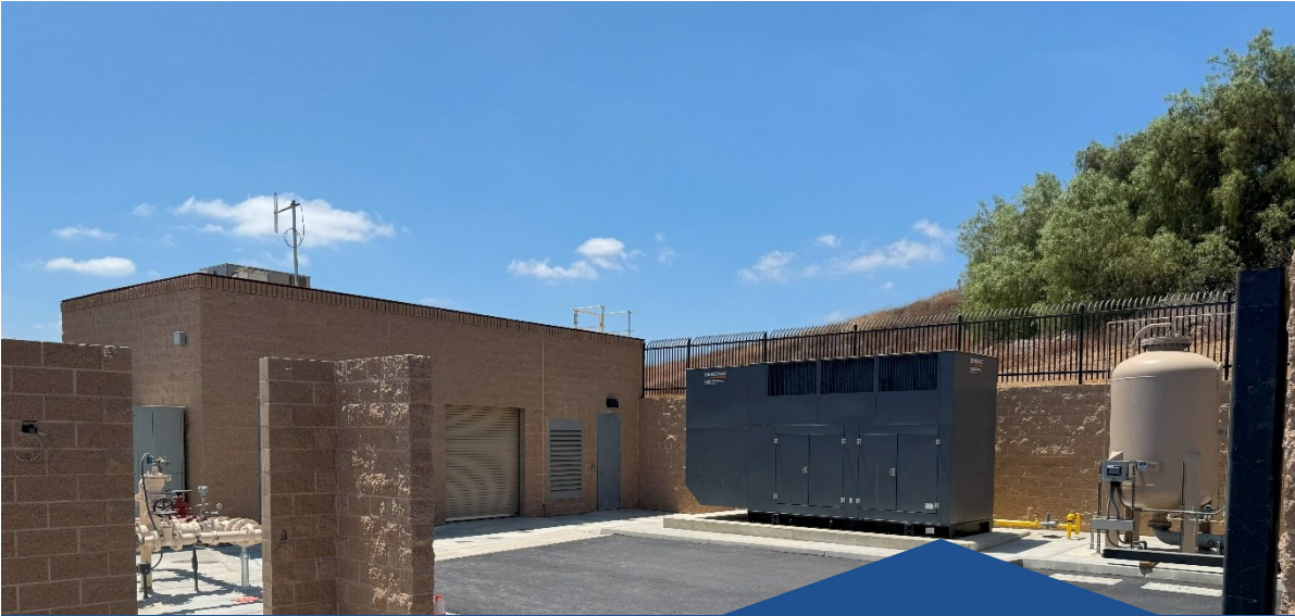
Timber Ridge B.P.S. Design Pumping Capacity: 2,700 GPM
