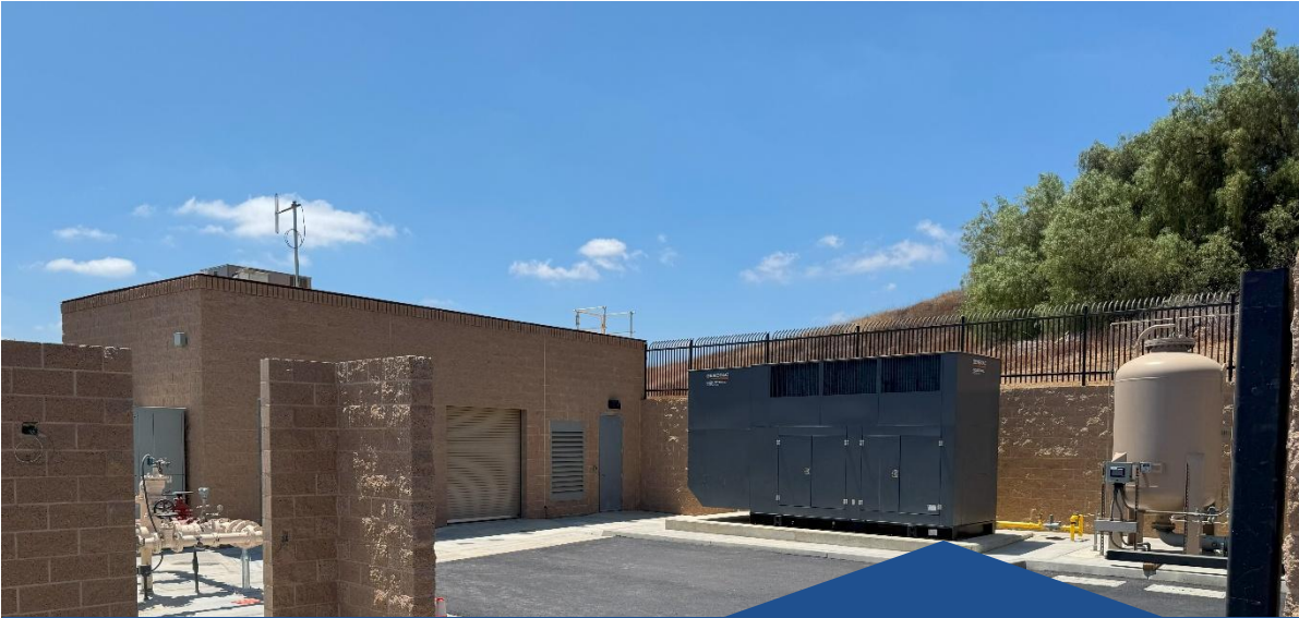
Timber Ridge B.P.S. Design Pumping Capacity: 2,700 GPM
