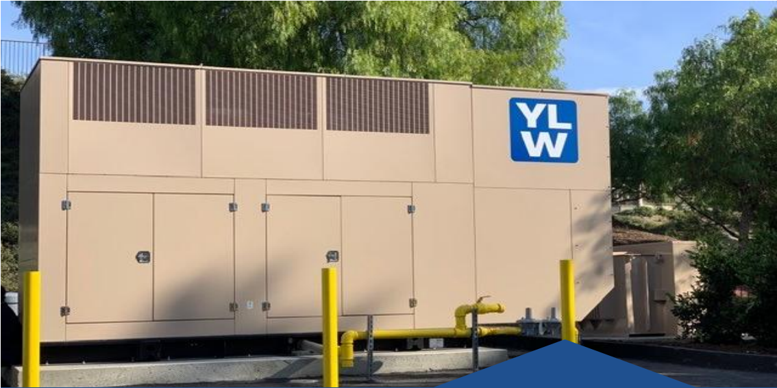
Elk Mountain Emergency Backup Generator – 500kw Elevation: 780'
