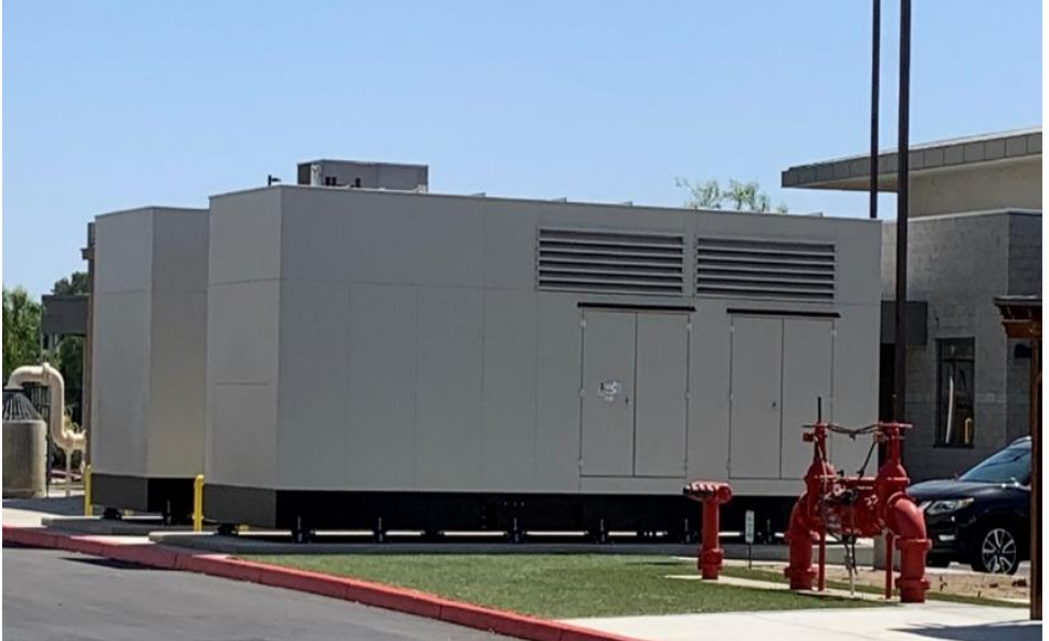
Emergency Backup Generators at YLWD Headquarters
